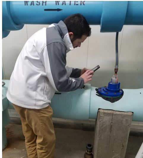
Staff checks a meter reading during a routine inspection.
