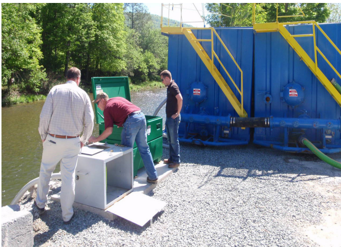
Staff inspects a surface water withdrawal intake and metering equipment.
